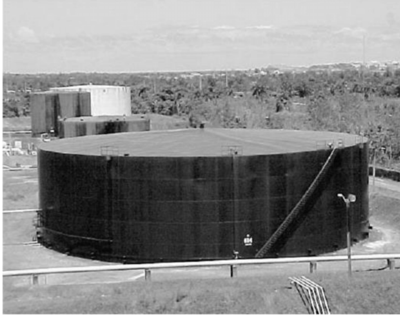
Figure 2. Image of the oil storage tank which is studied in this research.
